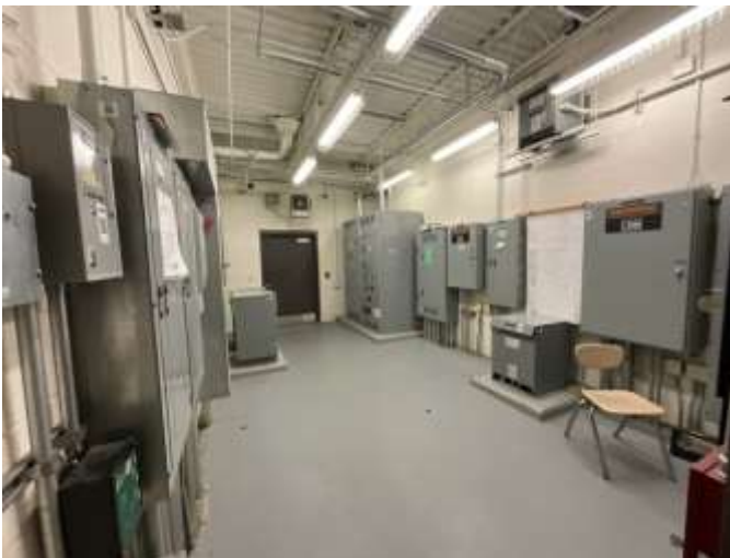
27 - MAIN ELECTRICAL ROOM
