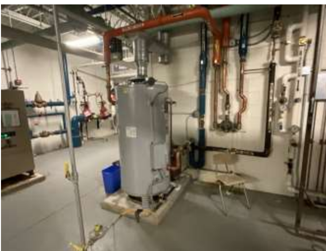
23 - DOMESTIC HOT WATER SUPPLY
