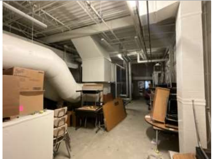
26 - SECONDARY MECHANICAL ROOM
