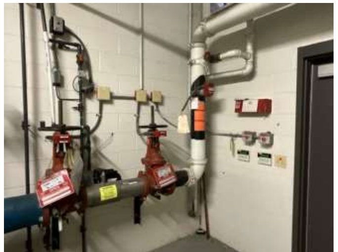
30 - FIRE PROTECTION ROOM
