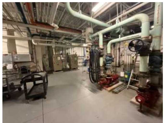
24 - MAIN MECHANICAL ROOM
