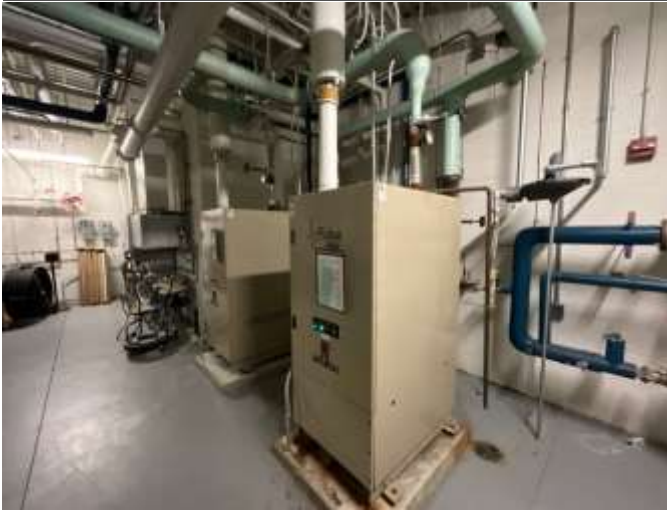
25 - BOILERS AND PUMPS
