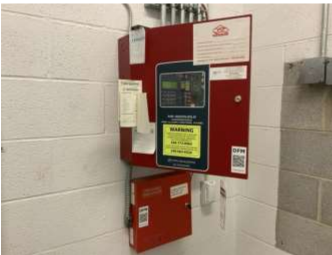
27 - FIRE ALARM PANEL
