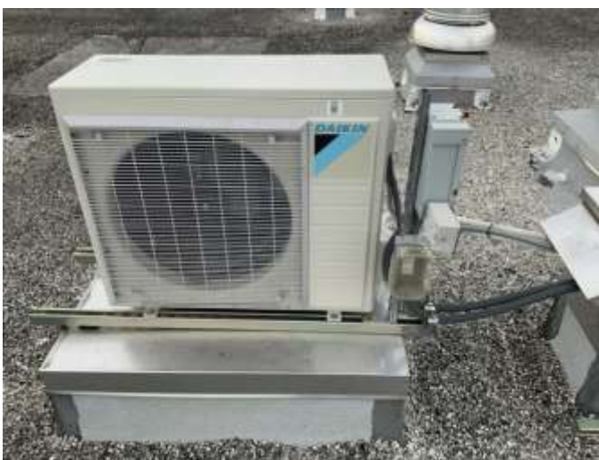
23 - SPLIT SYSTEM DUCTLESS
